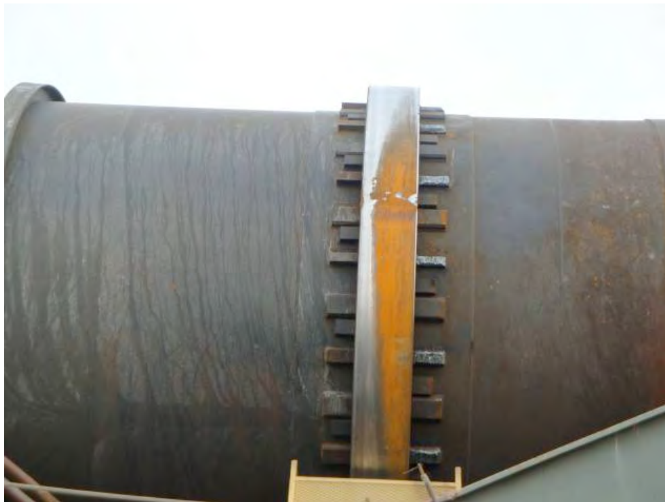
FIGURE 7 Heat-Stress Cracks in Trundle Caused by High Mix Temperatures for HMA RAP and RAS Mixtures
